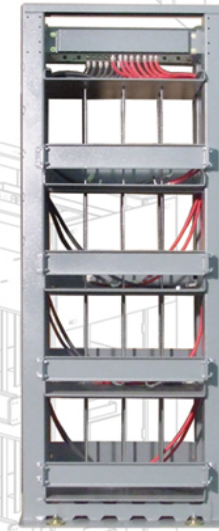
S045131 (24V) Welded Zone 4 / (4) Shelf (4) Wide
