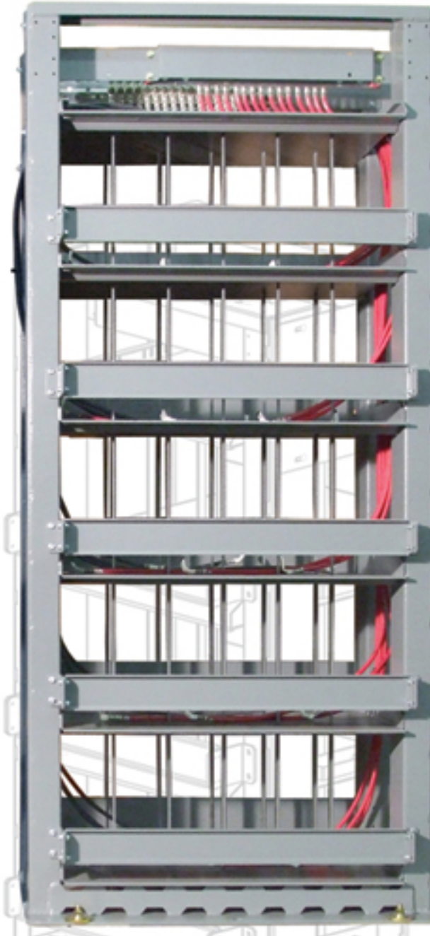
S046312 (24V) Welded Zone 4 / (5) Shelf (6) Wide
